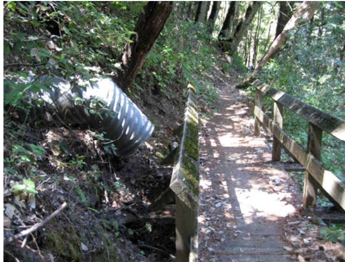
Photo 4: Storm water drain.
